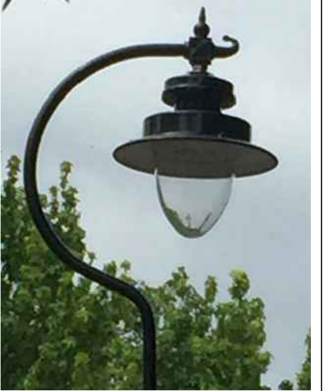
HERITAGE STYLE LED STREET LIGHTING IS TO BE USED (SUBJECT TO AGREEMENT WITH DfI-STREET LIGHTING)
